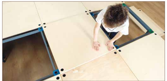
4. Lightweight decks are then placed onto the frame to form a robust structure, then bungs fill the frame holes.
